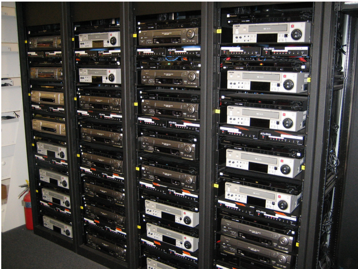
Figure 3. Media playback equipment rack (behind service desk).
